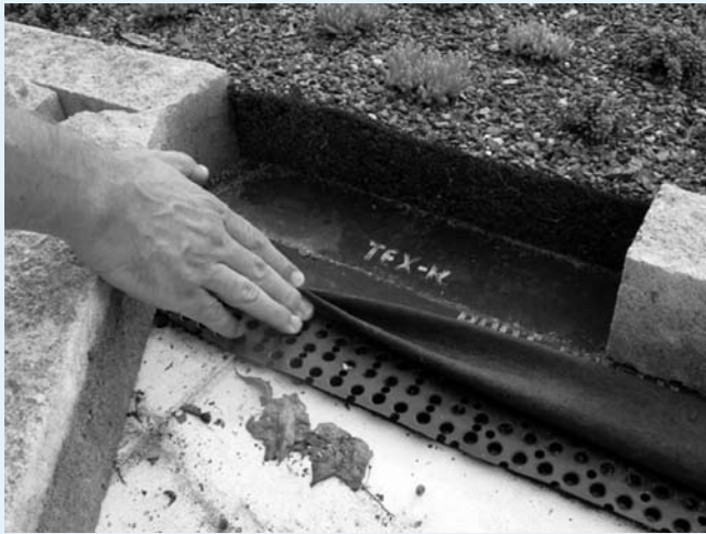
FIGURE 4. A cross-section of an extensive green roof shows storage “cups” in a drainage mat, 3 to 4 inches of an engineered soil media, and green roof vegetation overlying an impermeable membrane. (BAE, N.C. State University)
